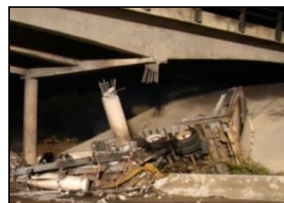
Figure 3: Impact damage of a bridge column
