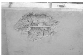
Figure 1. Typical local anchorage failure of slab
