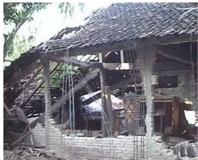
Figure 5. Javanese new culture house collapsed
