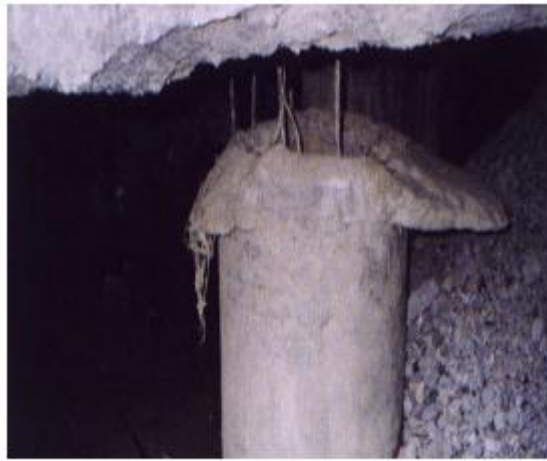
(a) Pile head released from pile cap due to inadequate detail connection
