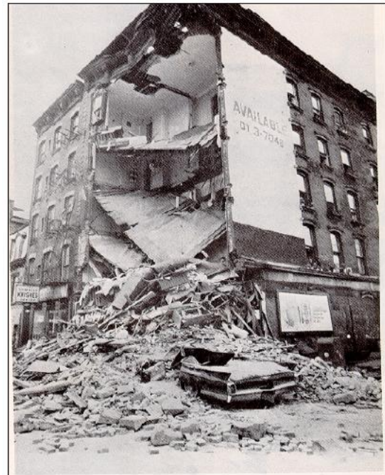
Figure 1. A building in New York after a vehicular collision (Allen and Schiever, 1972)
