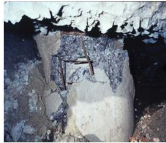
(b) Damage at pile head interface with pile cap
