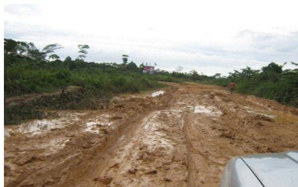
Figure 14. A bad-condition surface of road
