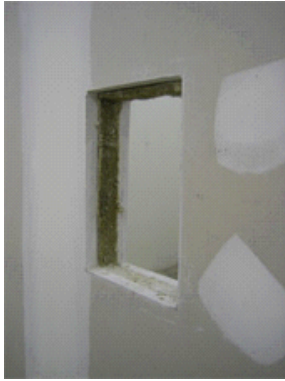
Figure 3a. Hole of dimension of 400 mm x 300mm was made on the existing filler wall (i.e. gypsum walls)
