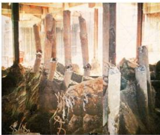
(c) Plastic hinges occurred within soil layers along pile height
