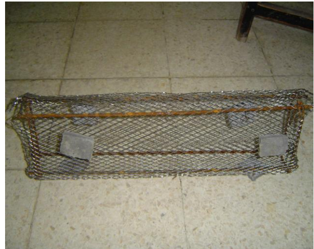
Figure 2. The placement of expanded metal sheet confinement for deep beams which cover the steel bar (Lelono and Widi, 2009; Susilorini, 2009a,b)
