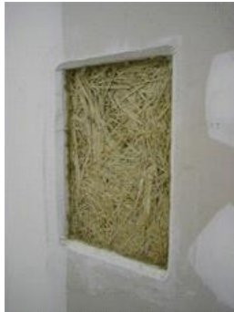
Figure 3b. Two layers of paddy-straws panels was put side by side, the tiny cavity gap between panels and wall were filled with rock wool floss to sealed it
